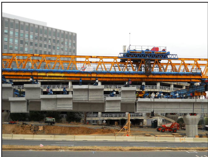
One of the two giant blue and yellow trusses is approaching the future Tysons West station causing overnight closures at Spring Hill Road through December. Closures will be announced as they are scheduled
