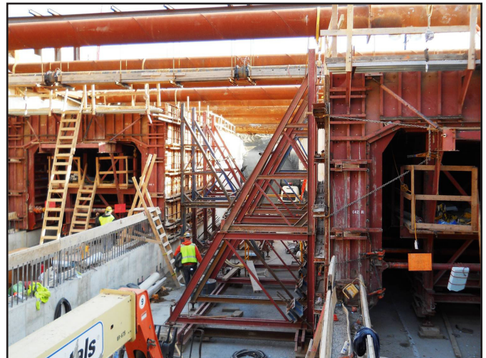
Dulles Corridor Metrorail Project crews have been working on tying in the new system with Metro's existing Orange Line.
